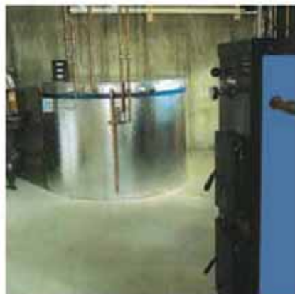
Excel boiler with Storage Tank.
